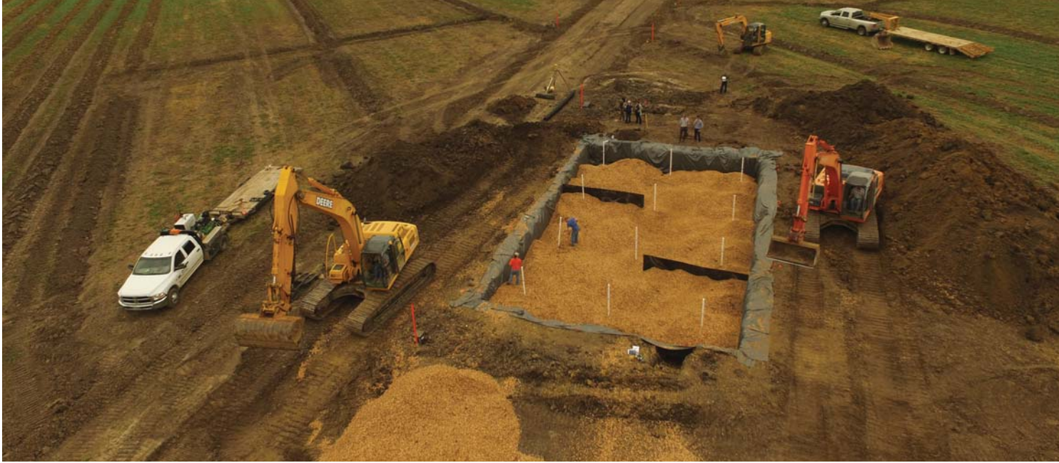
Aerial view of a woodchip denitrification bioreactor. Photo courtesy of Laura Christianson.
