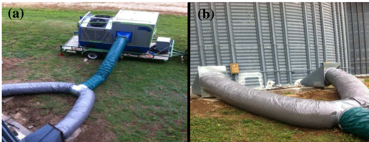
Figure 1. Grain chiller PCS-20 setup: a) Insulated duct connected to the chiller's outlet at one end and to a "T" connector at the other, b) Two ducts attached to the fan transition parts of the aeration fans that were removed.
