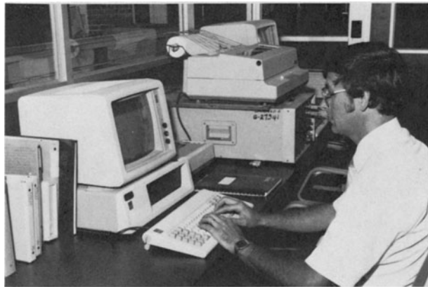
Figure 3. CUTIE SYSTEM EQUIPMENT AND CONTROL ROOM
