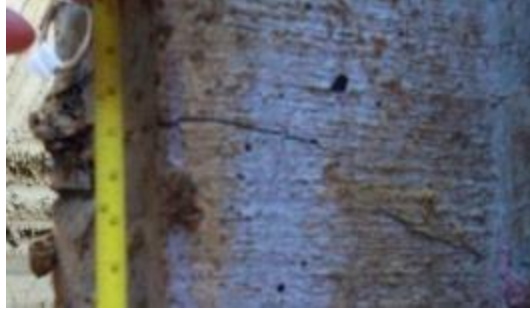
Fig. 18. A flexural crack found at a depth of 2.74 m below the top of P4
