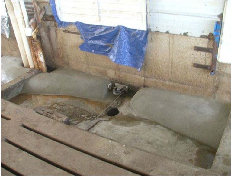
Photo 3. Concrete diverters used in the scraper system.
