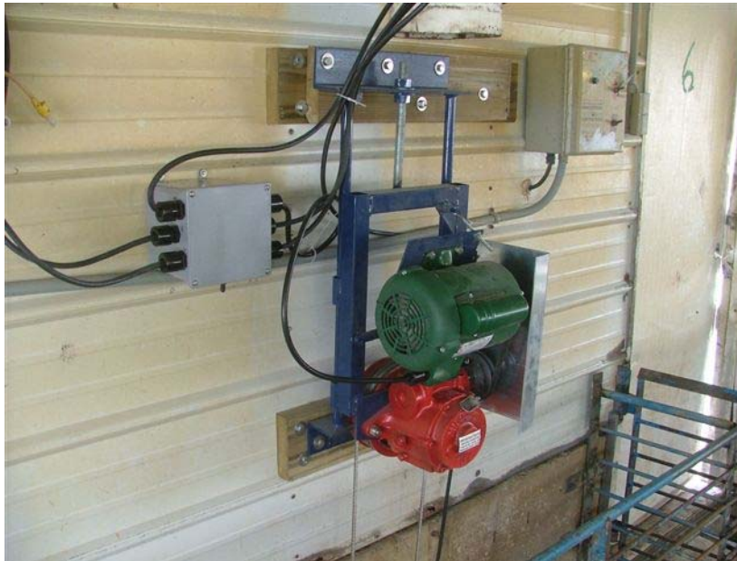
Photo 5. Safety features of the scraper system above the floor.
