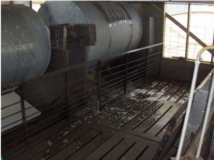
Photo 2. Flush tank has discharged its contents.
