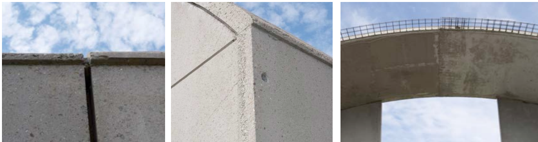
Figure 10A-10C: (Left to Right), Concrete broken at the roof edge, poorly crafted reveals at outside corner showing evidence of sandblasting on the surface, & a view of the underside of the roof showing the difference in quality in the concrete between the walls and the roof.
