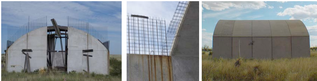
Figures 9A-9C: (Left to Right), The unfinished building with temporary bracing and roof panel formwork in place, the wall / roof intersection showing the modest reinforcing sizing, and a side elevation of the finished building showing sagging in the roof and deflection in end walls.
