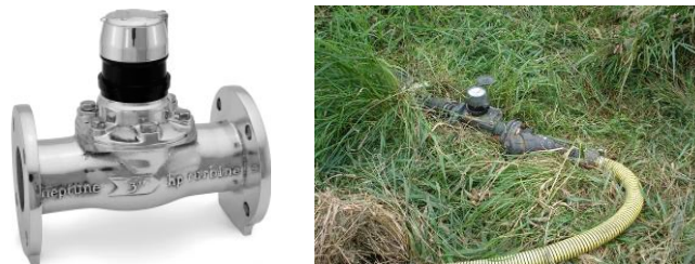
Figure 11. Neptune flow meter with Tricon/E3 encoder (left) and Neptune flow meter as installed to measure flow from the VIB into the VTA.
