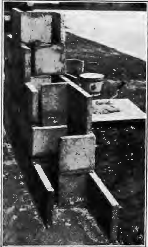
Fig. 14. There is little opportunity for the transmission of moisture or the conduction of heat in a wall laid up in this manner.
