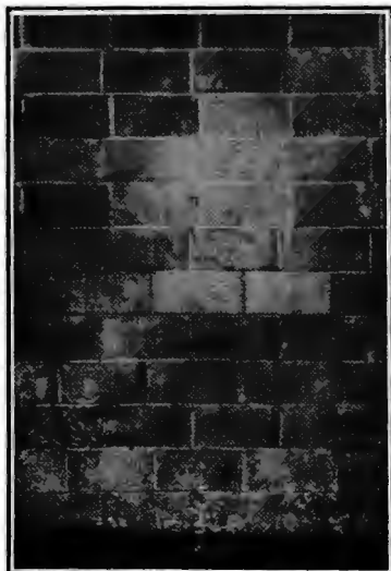
Fig. 13. The lower courses are double wall construction and the upper single wall construction.
