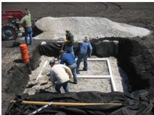
Members of the SFWA assisting in the installation of a blind inlet. In this image the drain pipe has been installed and connected to the riser and is being covered with gravel.
