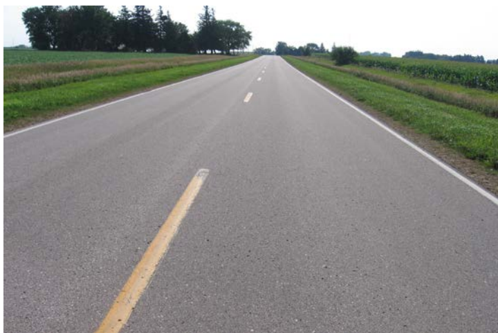
Fig. 4. Picture of distress-free HMA surface on rubblized PCC (test section no. 4: C23 in Franklin county)
