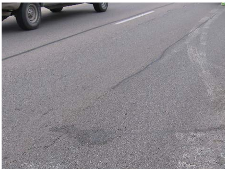
Fig. 5. Picture of Longitudinal crack on HMA surface over rubblized PCC (test section no. 6: IA141 in Polk county)
