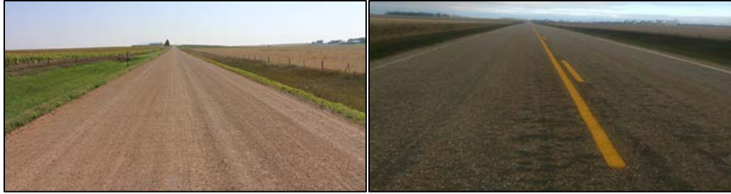
Figure 3. Appearance of Otta seal at immediately after the construction (left) and one month post construction (right).
