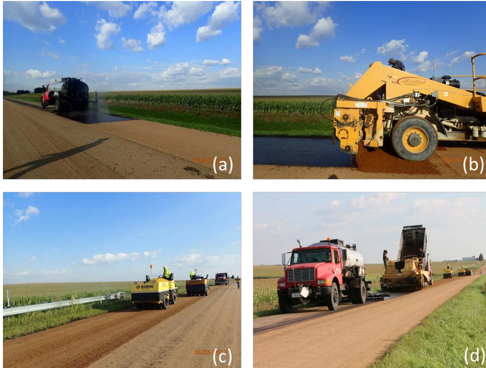
Figure 2. Otta seal construction process of (a) binder spraying, (b) aggregate application, (c) rolling compaction, and (d) the complete process.
