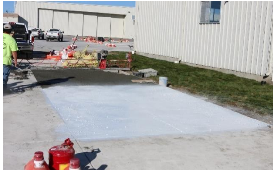
Figure 1. Construction of two ECON HPS test slabs at Des Moines International Airport, November 2016
