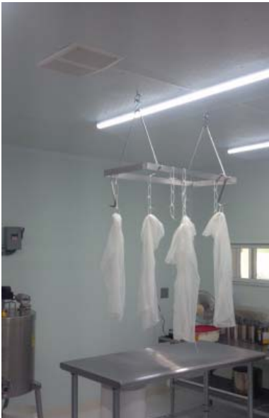
LED lighting in the Does and Divas Dairy processing building. The bags hanging from the rack are used to drain cheese in the processing room.
